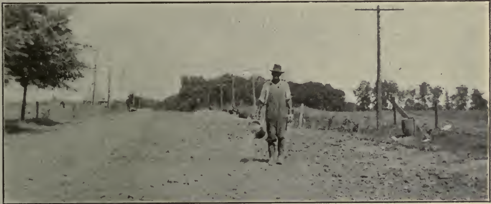
A PORTION OF ROUTE 5, ILLINOIS STATE HIGHWAY, BUILT BY McCALL CONSTRUCTION COMPANY, USING CALCIUM CHLORIDE FOR CURING
